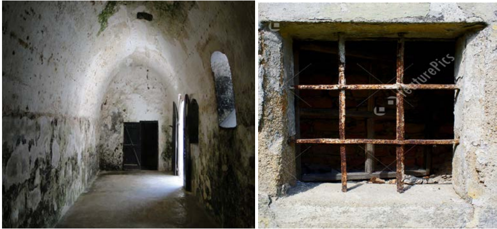
Fig. 3. Observations from Visual Inspection
