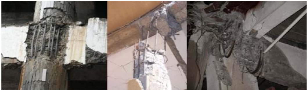
Fig.3. Failure Modes for Beam-Column Joint
